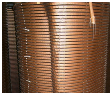
Buckling of winding
